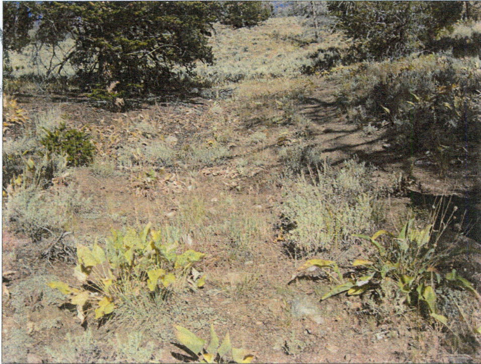
Photo Number 5: This is another portion of the access route in need of a water bar.
