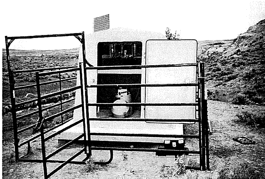
Figure 3. Streamflow gage on Pumpkin Creek. The equipment in the shelter records water levels in the stream, and also collects water samples when a flood occurs.
