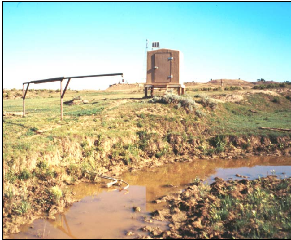
Figure 3.1-1. Continuous Record station at LX Bar Creek near Mouth consists of shelter containing automatic discharge and water sampling equipment, solar panels leading to inside battery storage, buried sampling lines to creek channel, staff gage in creek channel and on-shore cantilever stage-height gage (not included with every CR station).
